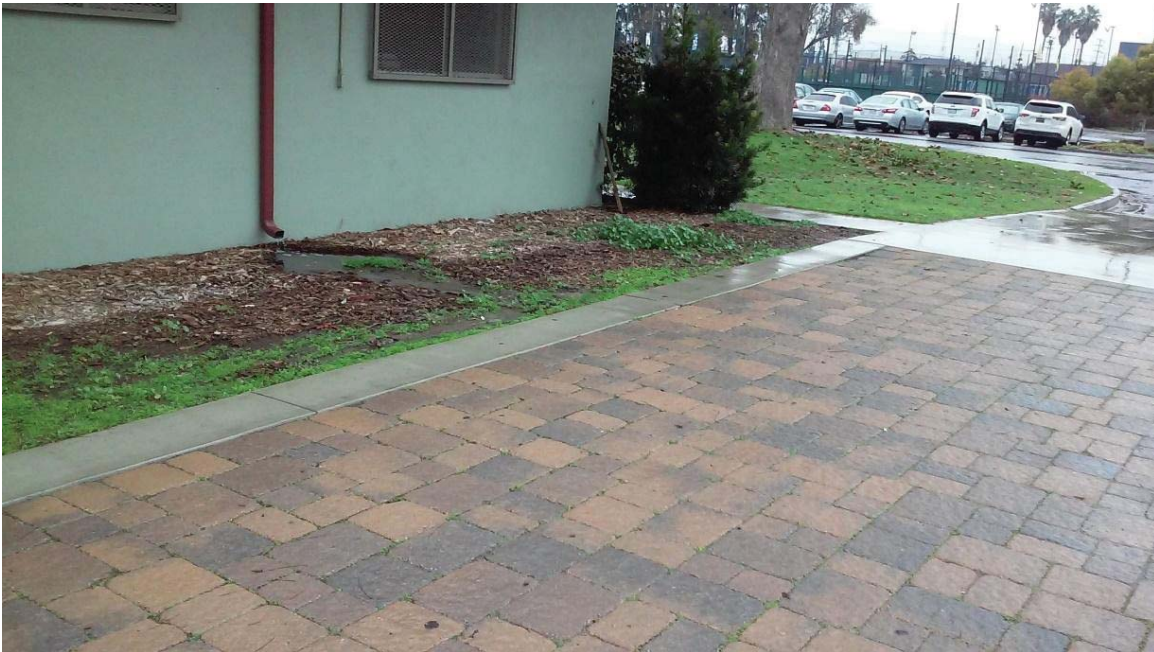
Figure 7: On the south side of the building water ponds on the Landscape area from the buildings storm water downspouts
