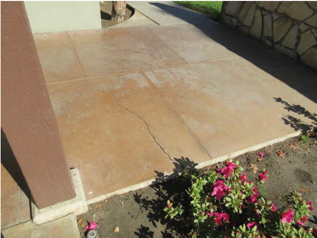
Photo 8 – Crack in slab on grade at front entrance.
