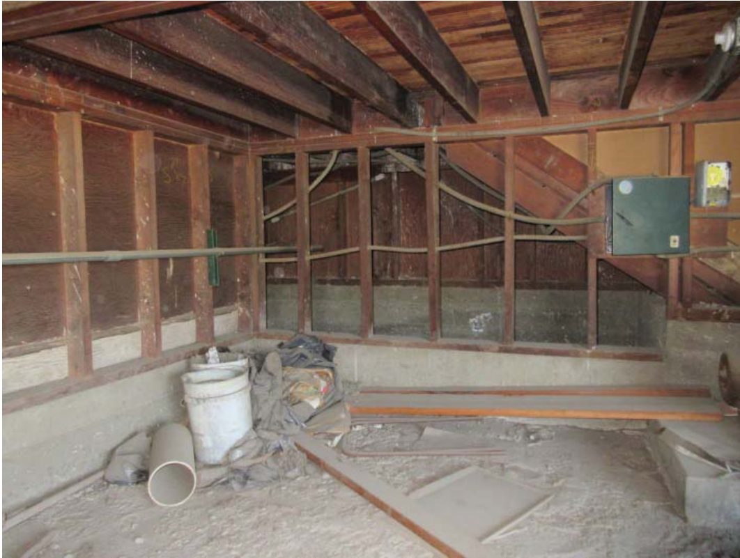
Photo 15 – South and east walls and wood framing below rear stage platform.
