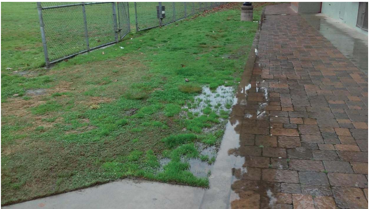
Figure 10: Ponding area in the back of the building where the walkway and landscape meet
