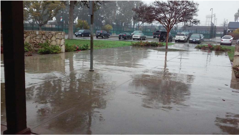
Figure 3: Front concrete walkway where there is no existing storm water drainage system
