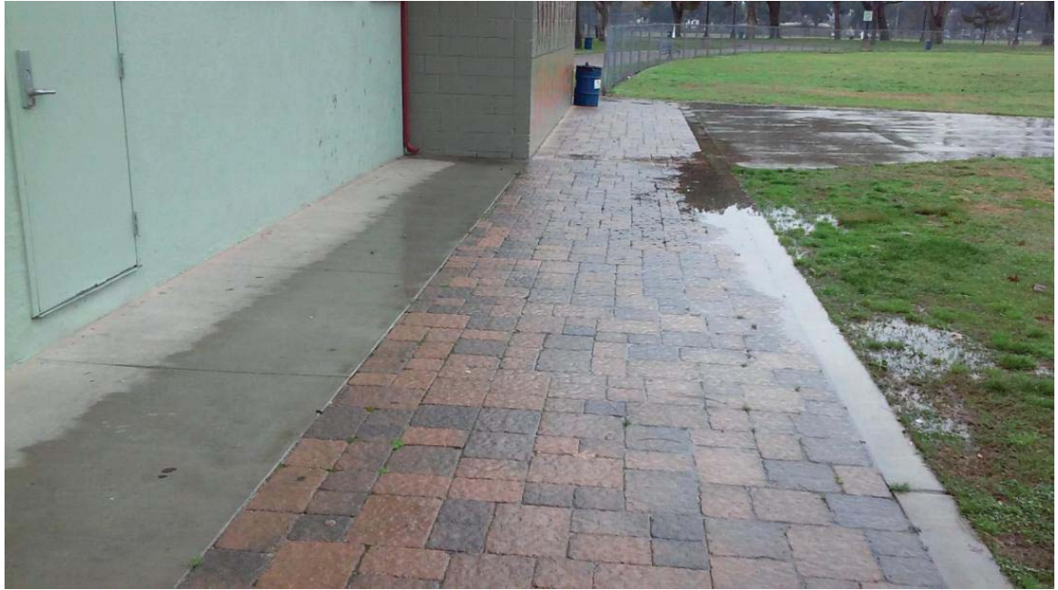
Figure 9: Water from downspouts flow into existing walkway in the back of the building
