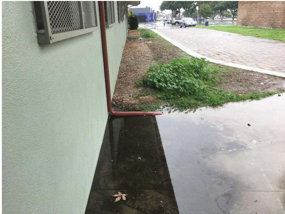
Figure 6: On the south side of the building water ponds on the concrete area from the buildings storm water
