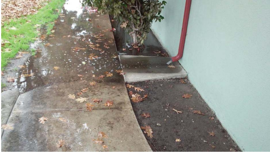
Figure 5: On the north side of the building water ponds on the walkway and partially flows back towards the building affecting the structural integrity of the building.
