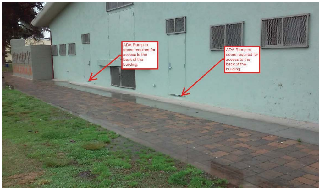
Figure 18: Non-compliant ADA accessibility in the back of existing building
