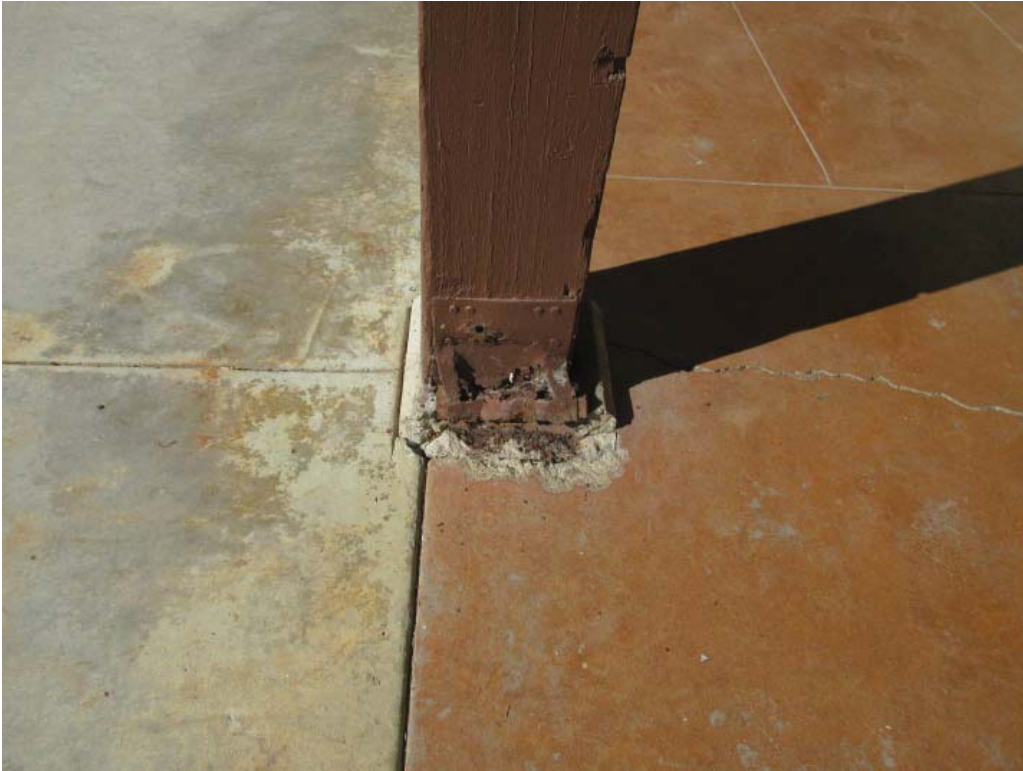
Photo 7 – Close up of Photo 6.
