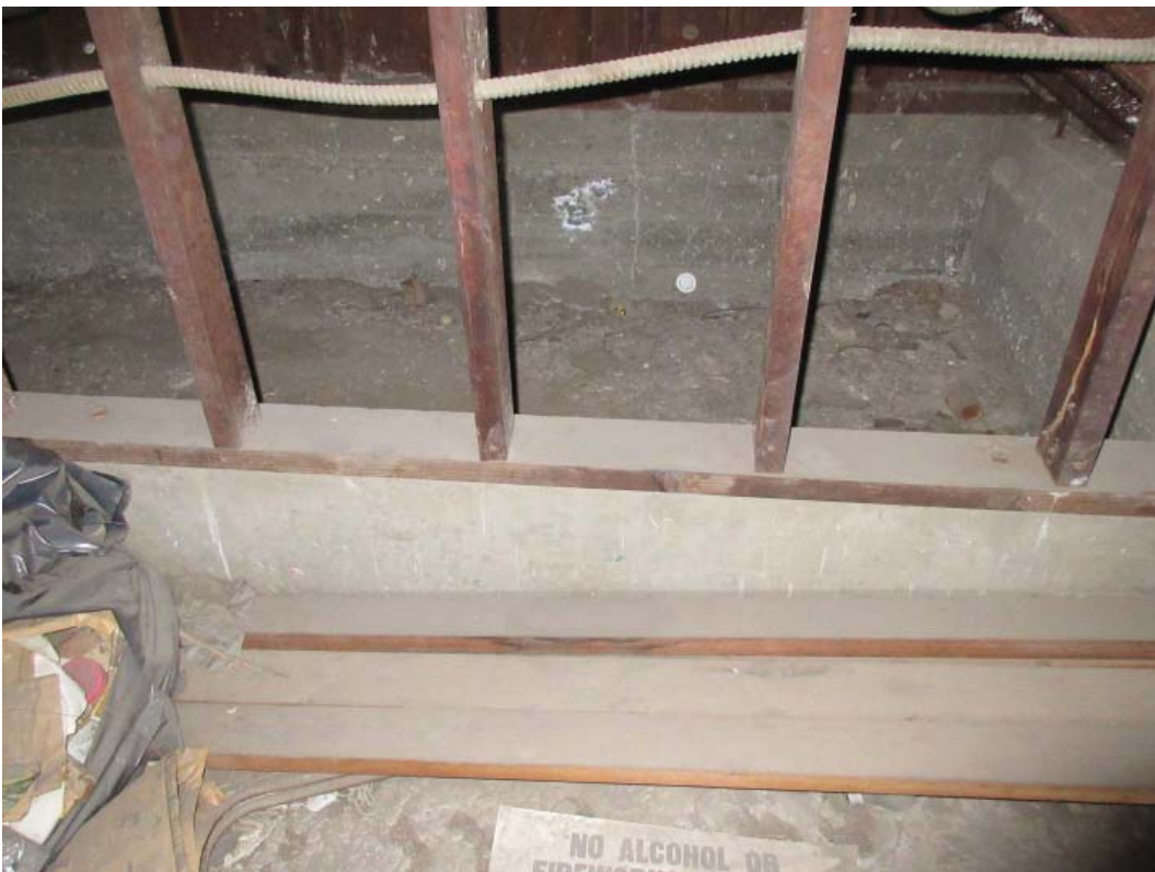
Photo 18 – Close up of north wall sill plates with anchor bolts, plywood, and stud framing below rear stage platform.
