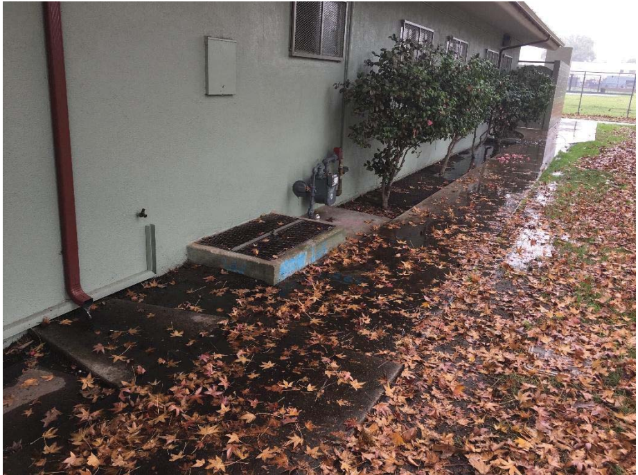
Figure 4: On the north of the Girls Club House storm water ponds on the walkway
