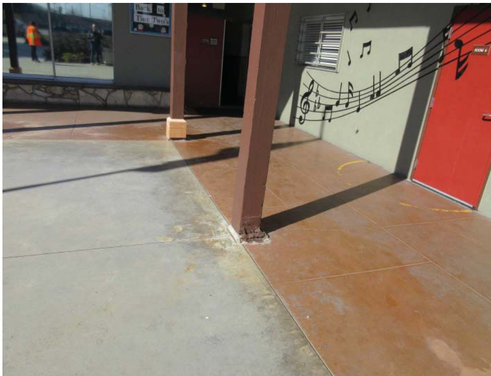
Photo 6 – Entrance wood framed colonnade column with deteriorated corroded base connection.
