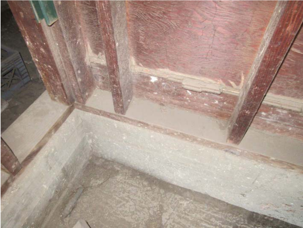
Photo 17 – Close up of north and east wall sill plates with anchor bolts, plywood, and stud framing below rear stage platform.
