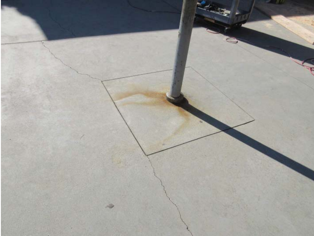
Photo 9 – Cracks in slab on grade near flag pole at front entrance,
